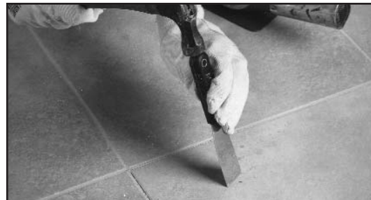
Fig. 28 - Drive a putty knife into the heated area and pry upward.
